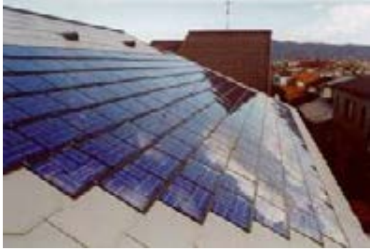
Figure 6 - Integrated photovoltaic panels
